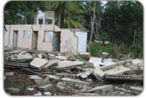
Destroyed school building in Kosgoda. More than two months after the tsunami hit, little has changed.
